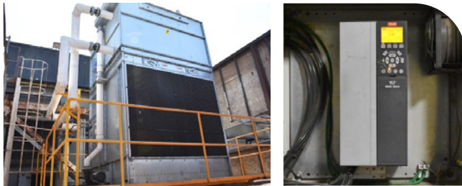
Installation of VFDs in Our Motors to Control the Cooling Tower
